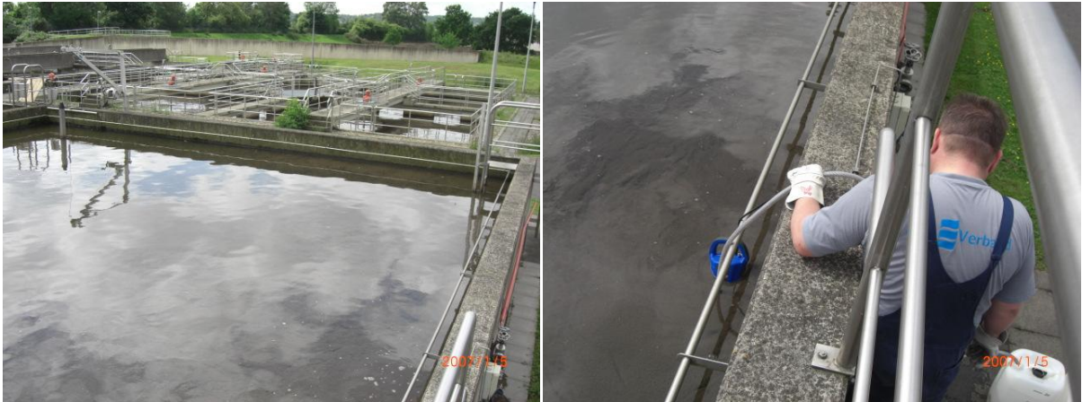
Figure 2-6. Denitrification tank (left) and wastewater sampling (right)
