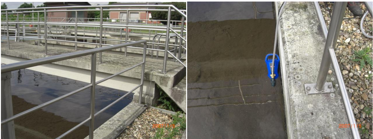
Figure 2-7. Bio-phosphorus tank (left) and wastewater sampling (right)
