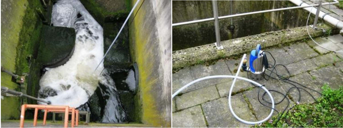
Figure 2-5. Discharge measurement well (left) located after secondary settlement tanks and water pump used for collection (right)
