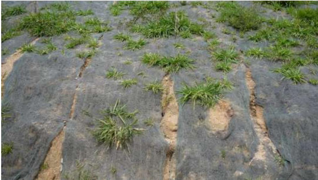
Figure 5: Geotextiles for initial slope stabilization on a roadside in Teresópolis (photo credit: Wolfram Lange)
