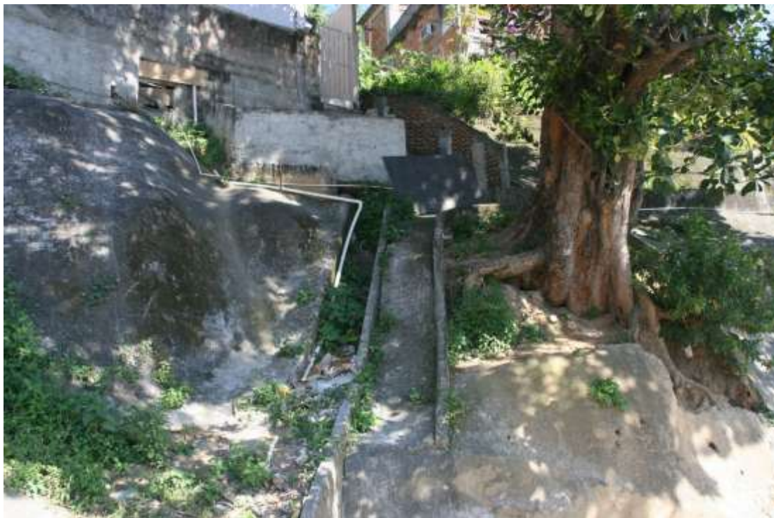
Figure 4: Protective structures with shotcrete, drainage pipes and drain ditch in an informal settlement in Rio de Janeiro (photo credit: Udo Nehren)
