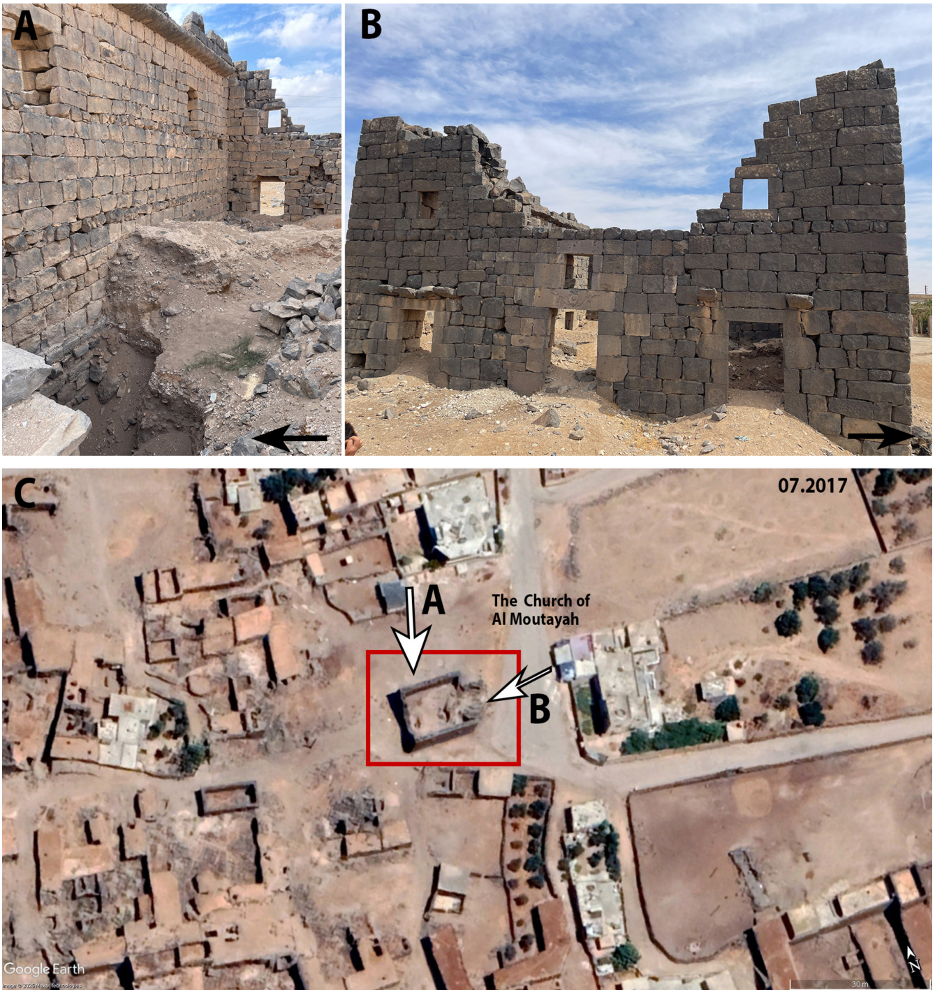
FIGURE 6 | (A and B) Looting pits documented in the church of Al Moutayah, extending beyond 2 m in depth, increase the likelihood of the wall collapsing in the future. The severity of this damage cannot be accurately assessed using satellite imagery alone, highlighting a key limitation of this method. (C) The church of Al Moutayah on satellite imagery in 07.2017 (Image 2025 Maxar Technologies. Used in accordance with the Google Maps/Earth terms of service for research purposes).
