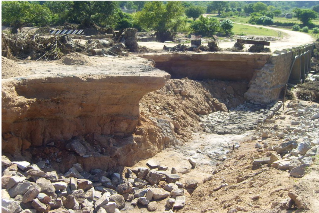
Figure 7. Broken bridge along Mwenezi river tributary
