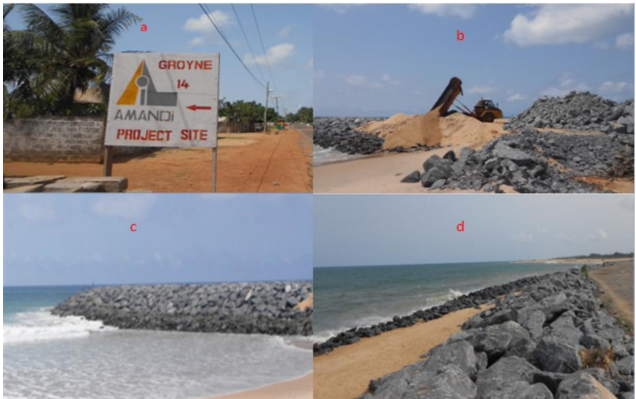
Fig. 9: Picture ‘a’ shows the construction site for 14 groins at Blekusu-Keta, picture ‘b’ shows some groynes being constructed at the time of the research, picture ‘c’ shows a groyne in Blekusu-Keta, and picture ‘d’ depicts a revetment in Keta Central. All pictures were taken during the fieldwork in 2019.
