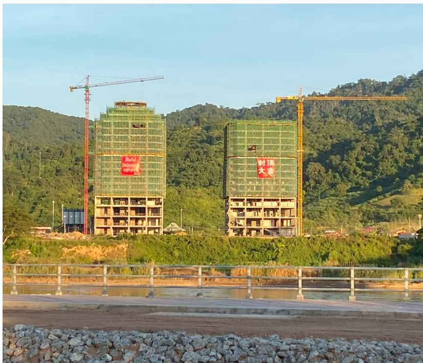
Figure 27. Two Buildings Invested in by Yunnan Hai Cheng Group on the Border of Huay Xai, Laos. October 31, 2019.
