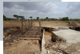
Spill-over blockages made out of cement allow the fresh water to flow during the rainy season, while blocking brackish water in the dry season. However, they are rare, might be 'left back' after the water found new ways and, in the absence of governmental maintenance, disintegrate. A bridge assembled out of sticks by the local communities allow for small transport and, with its localized malleability, contrasts the cement blockage.
